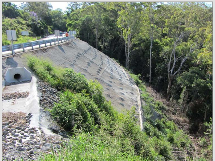
Right: Completed works on the Toowoomba Range crossing, Warrego Highway (Courtesy DTMR)
