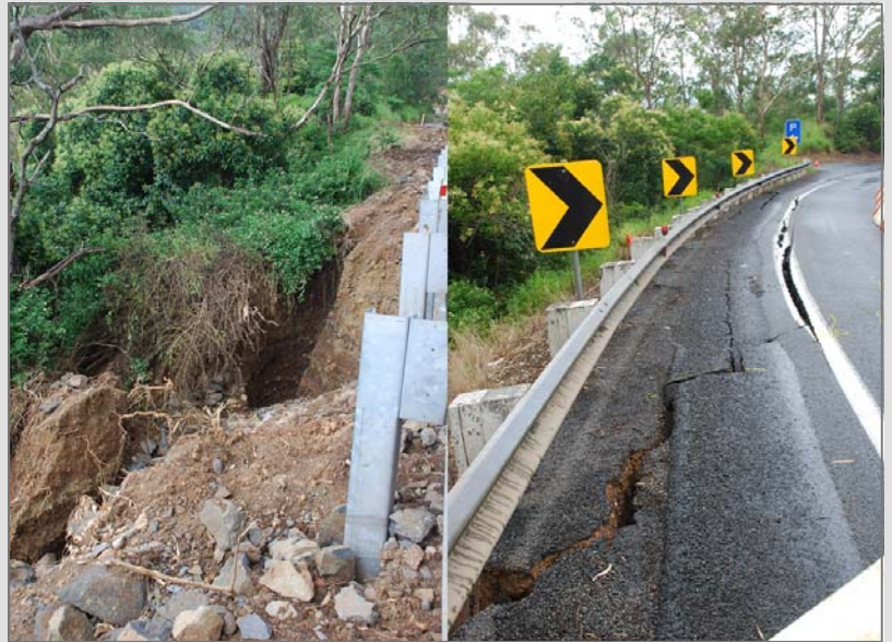
Image above shows damage to slopes and pavement on the Toowoomba Range crossing, Warrego Highway (Courtesy DTMR)
