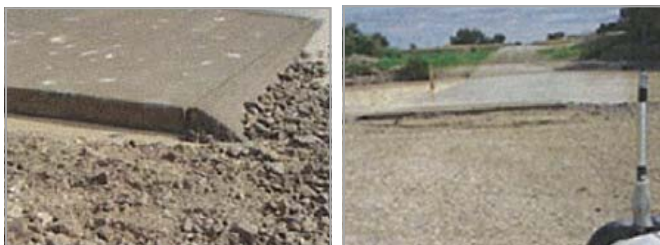
Above: Damaged sections at various locations on road at Stony Crossing.
