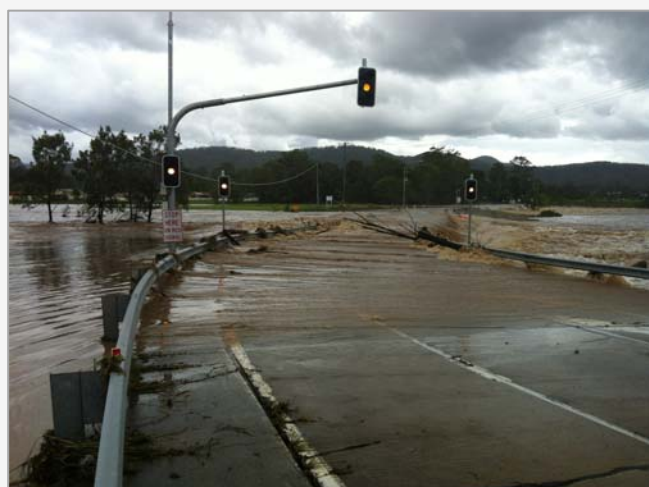
Above: The Coomera River in full flow again over the John Muntz Causeway in January 2013
