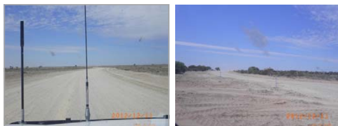
Above: Completed restoration works at various sections of road at Stony Crossing.
