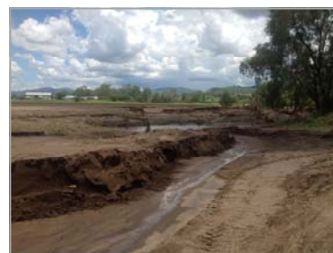
Above: Damage to Tenthill Creek and bridge.
