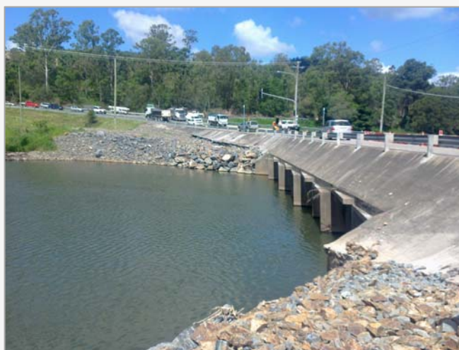
Above: John Muntz Causeway looking east, immediately prior to the start of construction, March 2013
