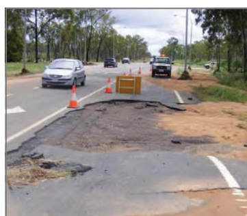
Peak Downs Highway – showing damage as a result of the 2010-11 events.
