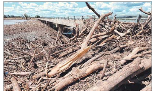
Above: Massive rainfall over the Burnett River catchment area resulted in this log jam at Mingo Crossing outside Bundaberg. (Courtesy Courier Mail, 7 February 2013).
