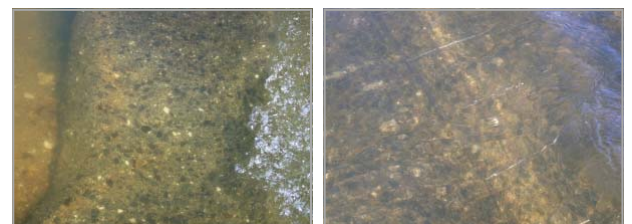
Images taken through water showing edge washed away (left) and exposed mesh and turbulence caused by hole in slab (right).
