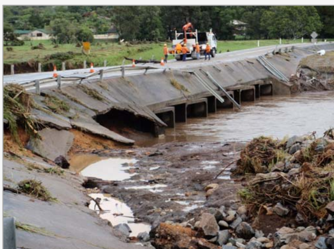
Above: Damage to the John Muntz Causeway after the Coomera River flooded in January 2010
