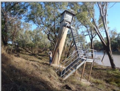
Gauging Station at St George after flood damage
