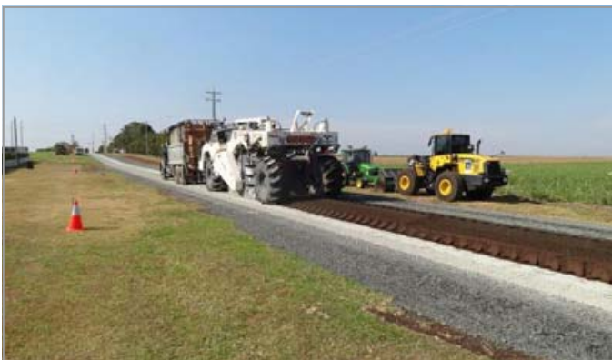
Photo above: In situ stabilisation of Hummock Road. Complementary works in Bundaberg deliver value-for-money outcomes.
