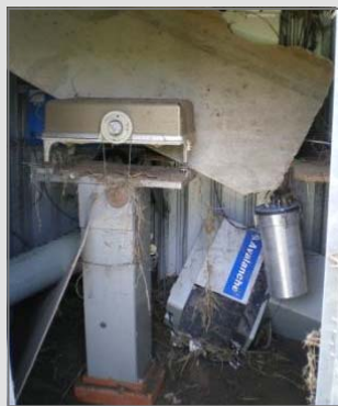
At left: Brisbane Valley gauging station hut - site after flood damage
