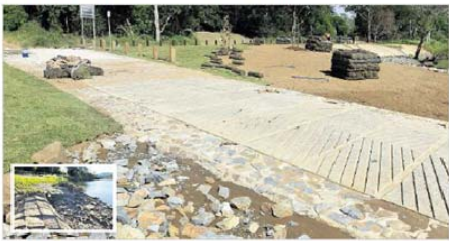
ABOVE: RECENT rebuilding of Riverside Park in Karilee is nearing completion after a flood destroyed the park including the boat ramp. RIGHT: Plan of the new work.
