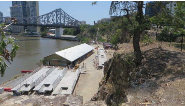
Looking down at the pre-cast girders being stored at Howard Smith Wharves
