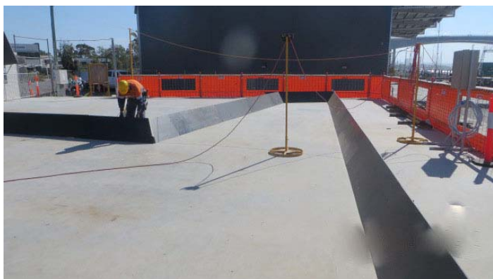
Getting ready to cast one of three special irregularly shaped deck pieces to accommodate the rest area and angles of bends along the zig zag alignment of Riverwalk.
