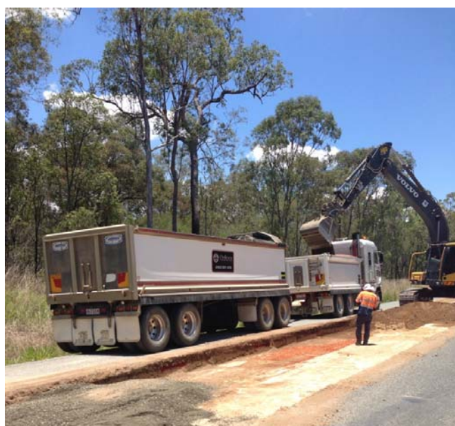
Above: patching works underway on Bruce Highway, north of Miriam Vale – December 2013
