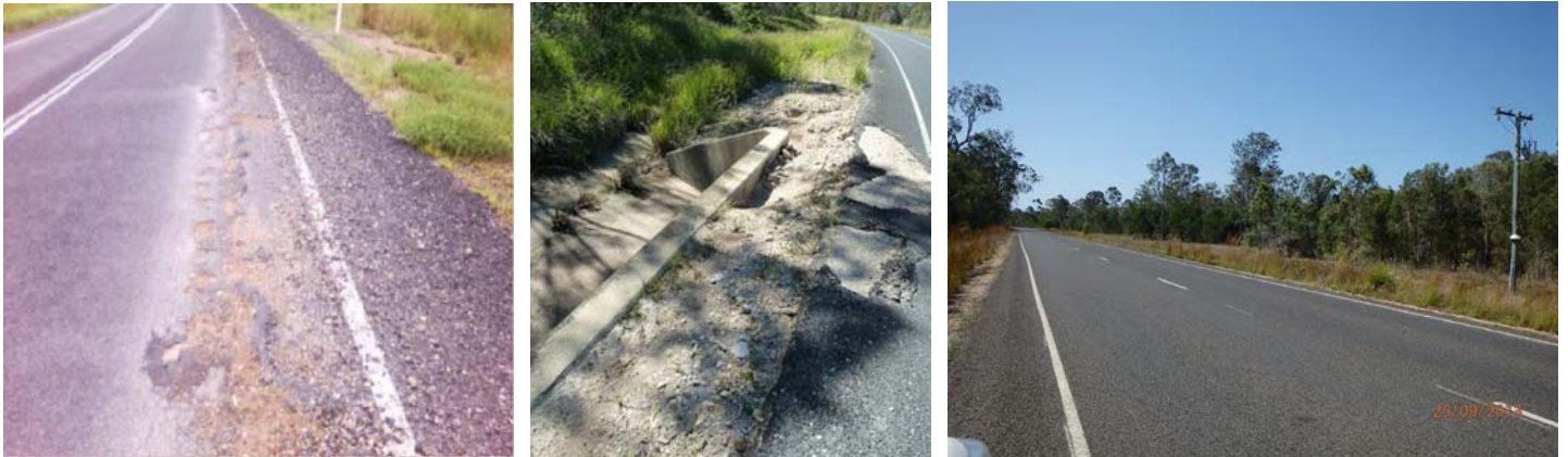
Above: damage to Round Hill Road following the 2011 flood event (left and centre); and following reconstruction works (right)
