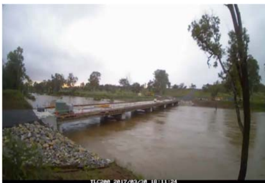
Above: Burnett River Bridge – ex-STC Debbie flooding of sidetrack and in Burnett River
