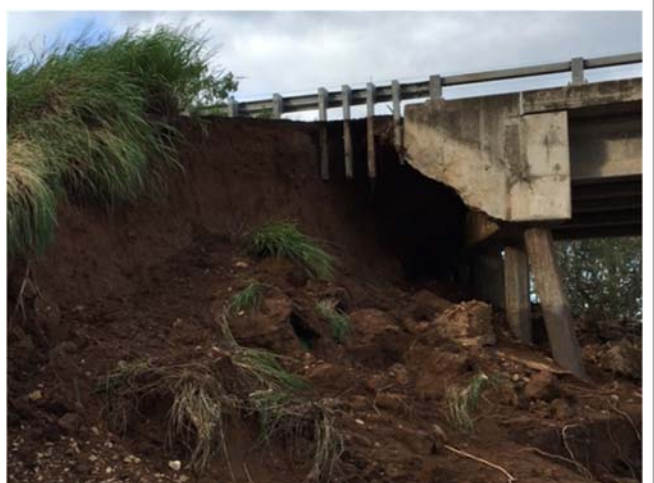
Damage to State road assets by Severe Tropical Cyclone Debbie. From top: John Muntz Causeway, Gold Coast; Pine Creek Road; Sarina Range- (Marlborough-Sarina Rd) Granite Creek Bridge (Bruce Highway)
