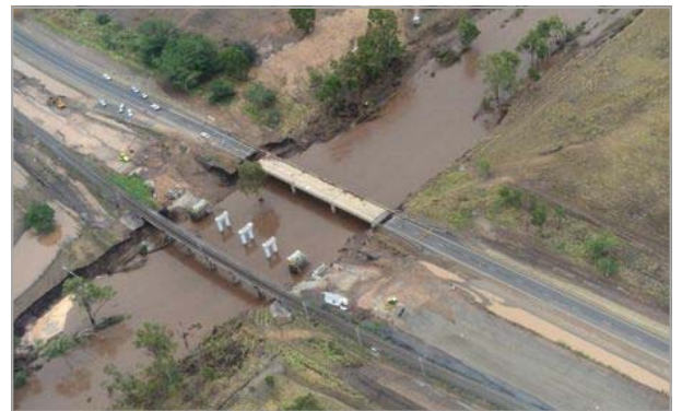
Damage to Capricorn Highway at Neerkol Creek, January 2013 (Courtesy www.themorningbulletin.com.au ).
