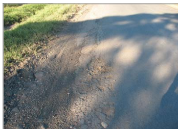
Above: showing damage to sections of Craignish Road.
