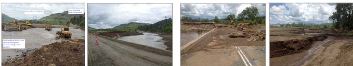
Above: Showing the impact to Hahns Crossing (left) and near re-opening (right) - March 2013
