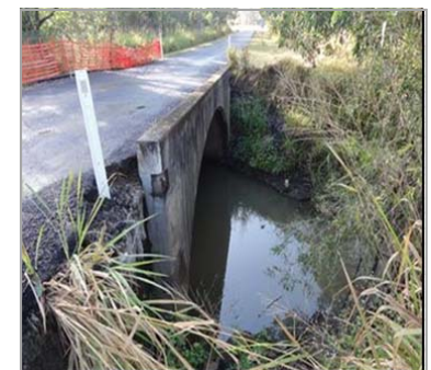
Above: showing damage to Gentle Annie Bridge in 2011.
