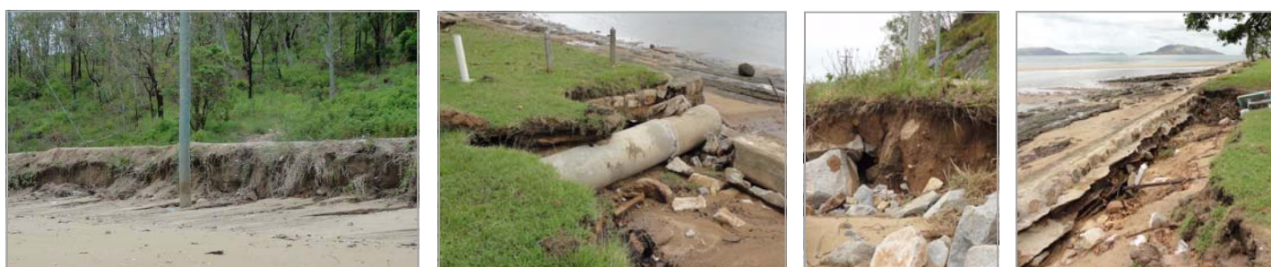
Images above showing damage to sections of Palm Island the seawall following Tropical Cyclone Yasi.
