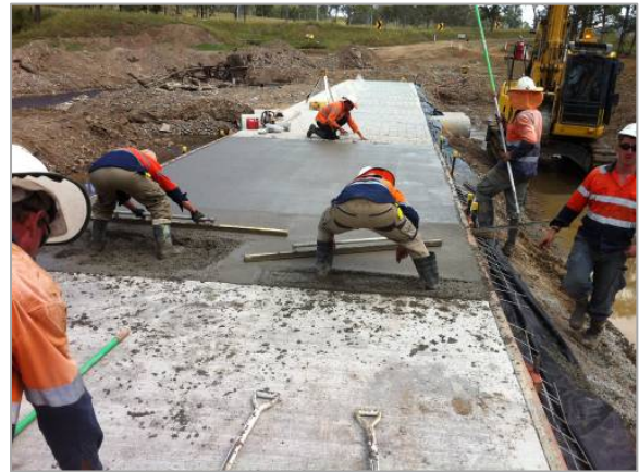
Above: recovery works in progress (March 2013) on a section of Gladstone-Monto Road.
