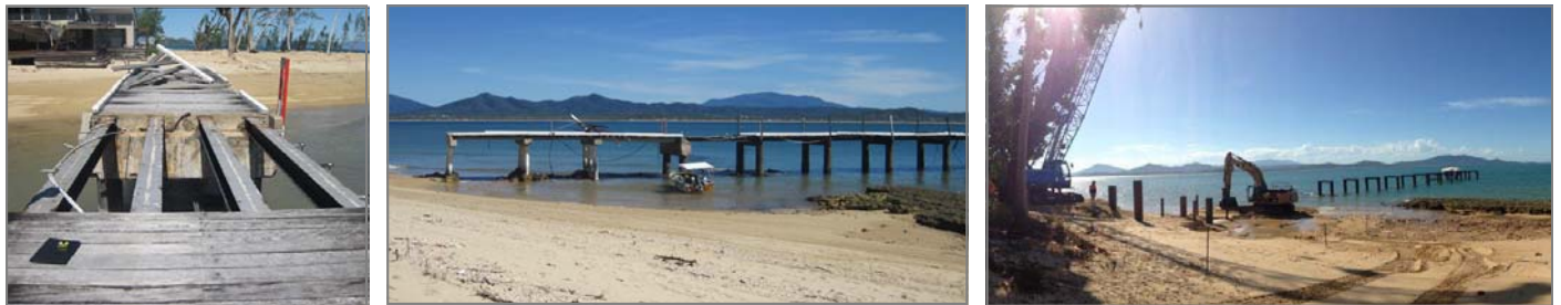
Above: showing extent of damage to Dunk Island jetty following Tropical Cyclone Yasi in 2011 and during reconstruction (on right).
