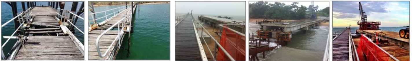
Above: showing extent of damage to Clump Point jetty.
