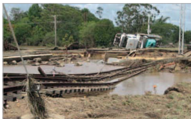
Above: Track damage - North Bundaberg (Image courtesy www.queenslandrail.com.au)
