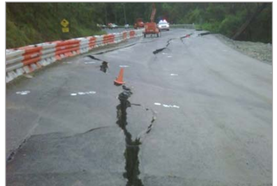
Above: Cunningham's Gap damage January 2011.
