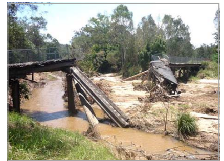
Above : The former Esk pedestrian bridge - after the flood, January 2011
