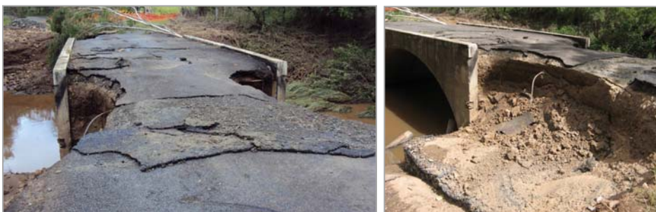
Above: showing extent of redamage to Gentle Annie Bridge in January 2013.
