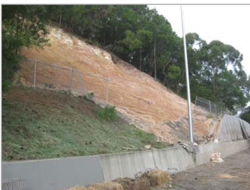
Photos at left and right show Tugun Bypass with landslips above the road in 2011.
