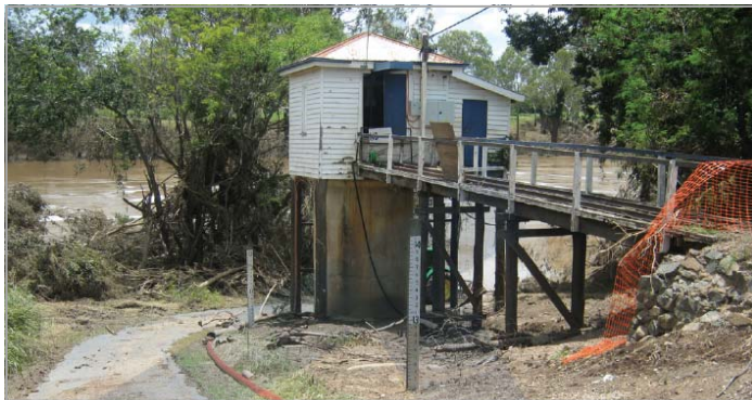
Above: Gayndah Water Intake Plant damaged in 2011.
