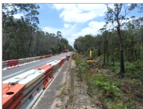
Above: Reconstruction works were able to start to remediate the slope and the pavement.
