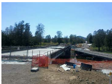
Right: construction works Grigor Bridge, November 2013— view looking towards Conondale (left); and finishing operations at both infill slabs (right)
