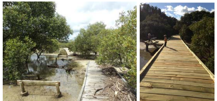
Above: damage (left) and post-completion (right) to the Berree-Badalla boardwalk
