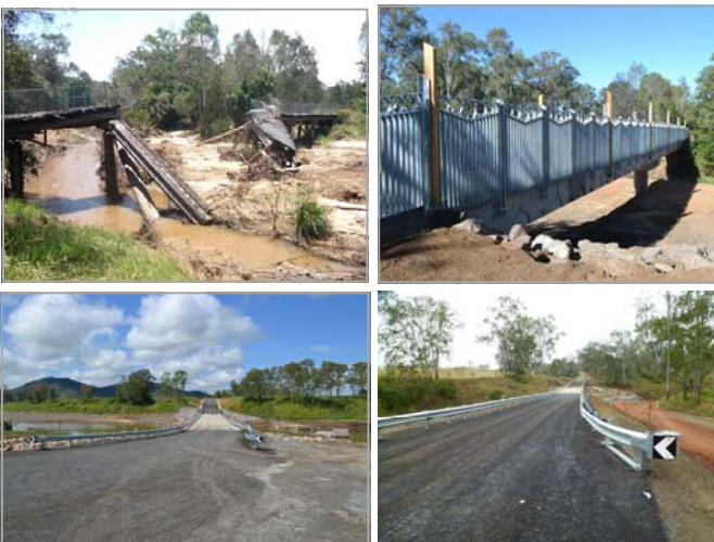
Top: Esk Pedestrian Bridge—damage (left) and following reconstruction (right) Below: Completed works at George Bishop Bridge (left) and Alf Williams Bridge (right), Somerset Regional Council
