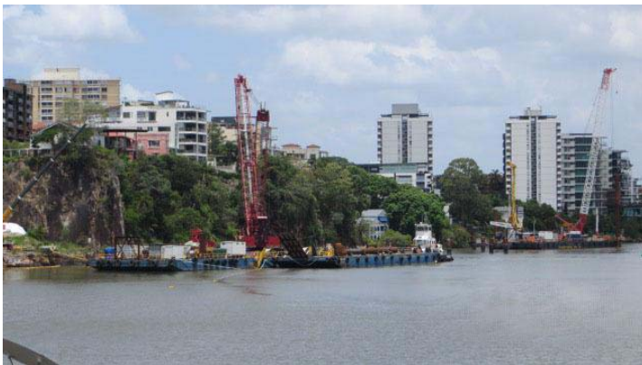
Left: Arrival of the barge that will be used to place the pre-cast concrete girders
