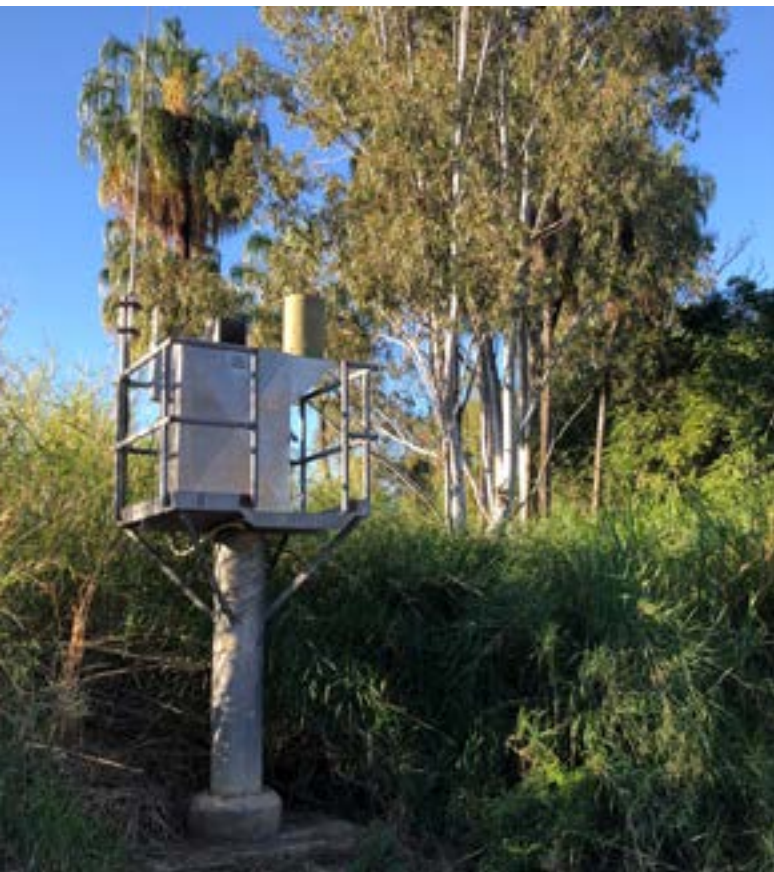
Image (above): Burdekin weir. (Left:) Automatic flood warning gauge at the Giru rail bridge.
