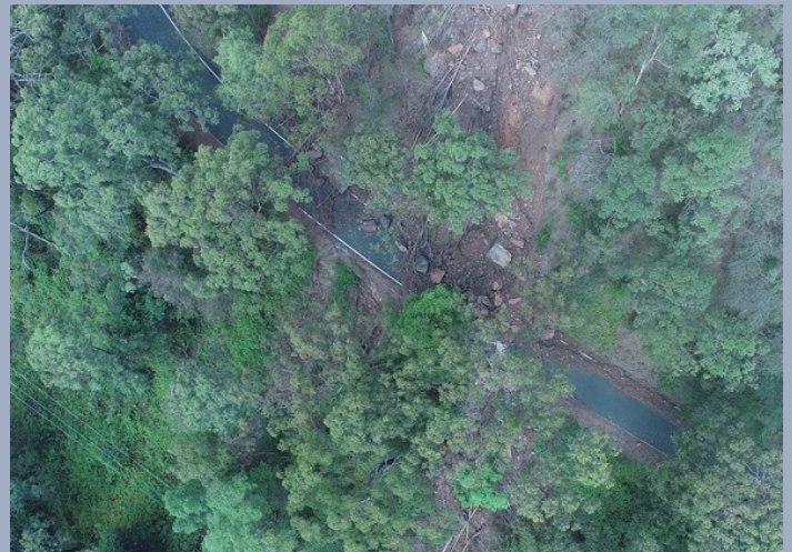
Image: Tamborine Mountain Road – damage site.
