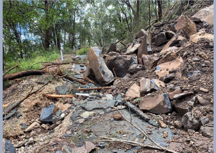
Image: Tamborine Mountain Road – landslide on road.
