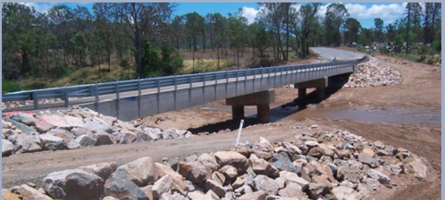
Images: George Bell Crossing washed away in January 2013 (top) and rebuilt with Betterment in 2015 (below).
