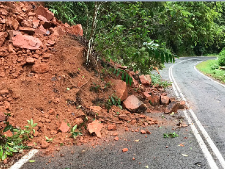
Image: Gold Coast–Springbrook Road – landslip following SEQ Rainfall and Flooding event (February 2022).
