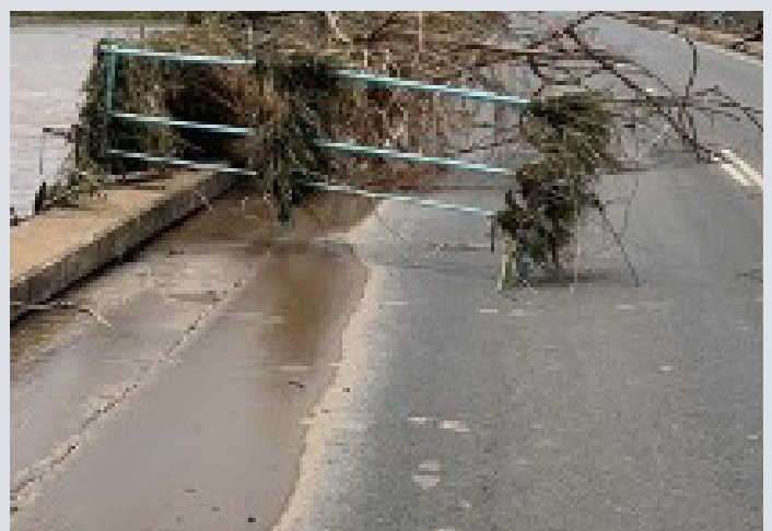
Lamington Bridge – damaged upstream handrails
