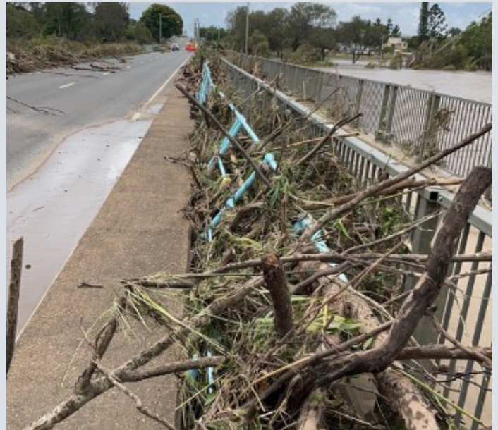
Lamington Bridge – damaged downstream handrails
