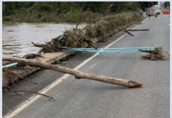
Lamington Bridge – damaged upstream handrails
