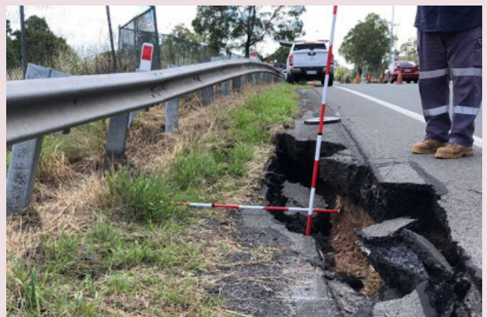
Brisbane Road – crack in road requiring lane closure (March 2022)
