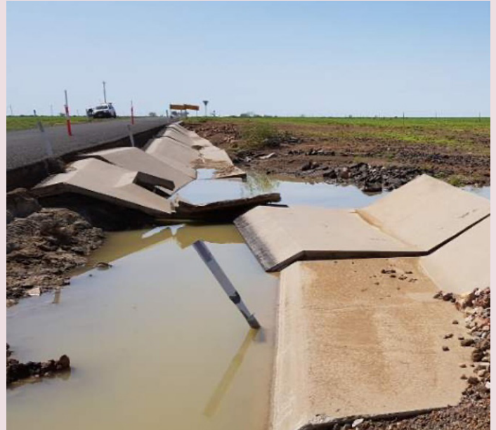
Muttaborra–Aramac Road – damage from Queensland Monsoonal Flooding (February 2020)
