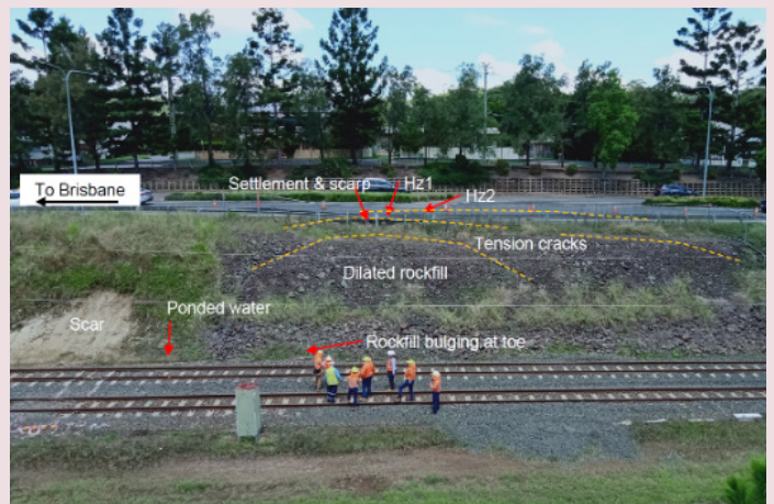
Brisbane Road – damaged area showing the slip, cracks and rocks at the embankment
