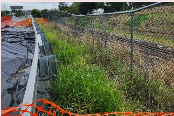
Brisbane Road – rail corridor running alongside the road at the damage site
