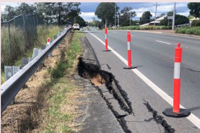
Brisbane Road – part of the 800mm deep crack, next to the road (February 2022)
