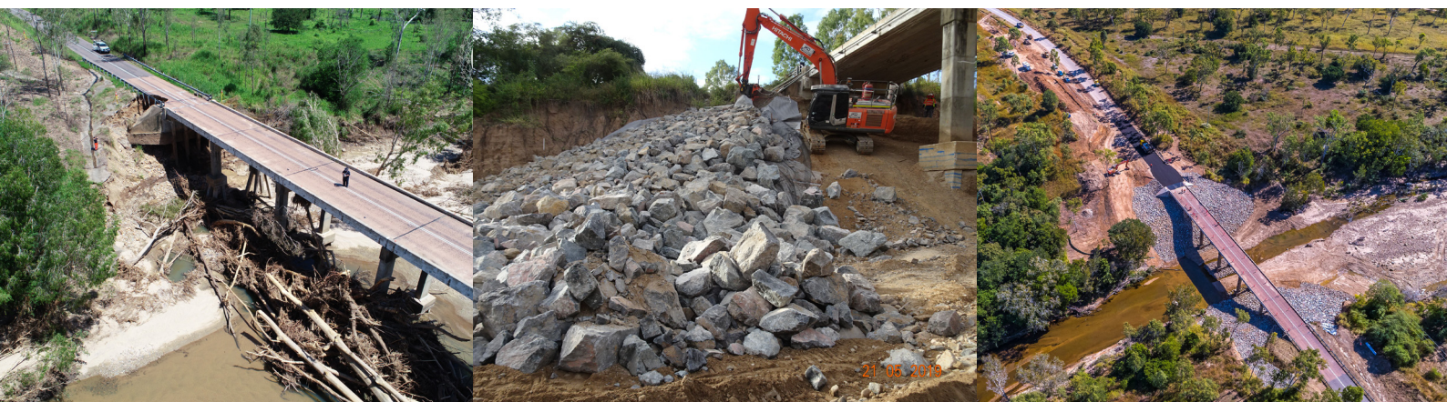
Image (l-r): Damage to Alice River Bridge from the North & Far North Queensland Monsoon Trough (25 January - 14 February 2019), reconstruction process, aerial view completed works.
