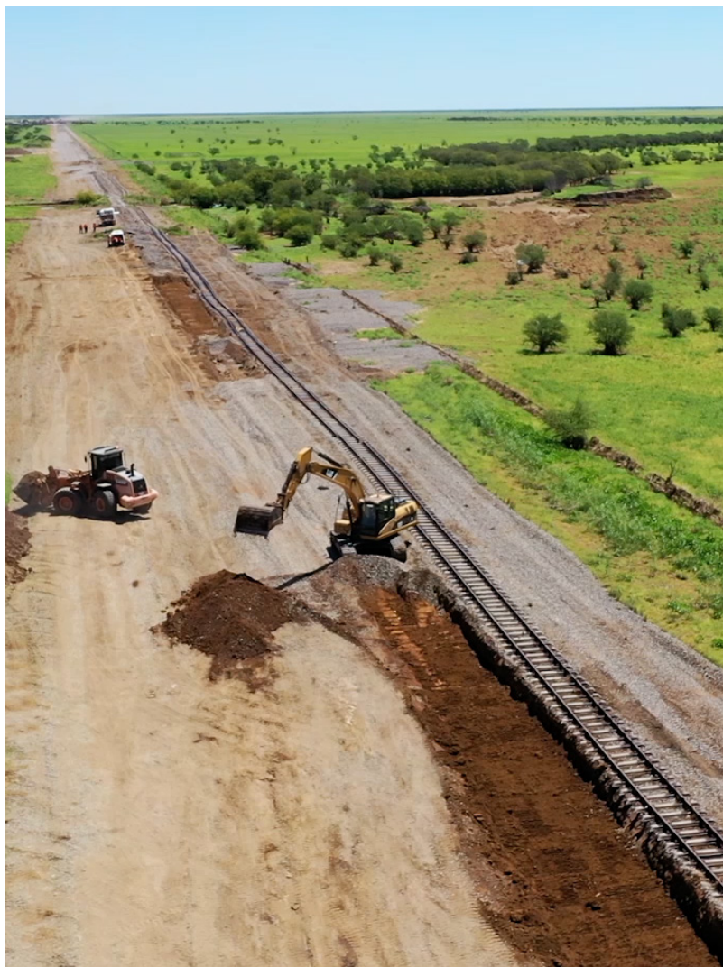
Image: Repair works to Mount Isa rail line following damage during the 2019 North & Far North Queensland Monsoon Trough.
