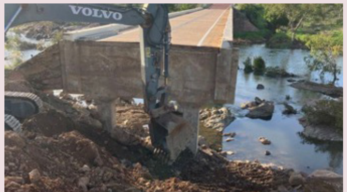
Gulf Developmental Road at Routh Creek Bridge – emergency works to remove the damaged embankment at the eastern abutment (January 2024)
