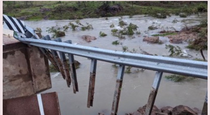
Gulf Developmental Road at Routh Creek Bridge – damage from North Queensland Monsoon Trough in January 2024 (Image: Queensland Police Service)
