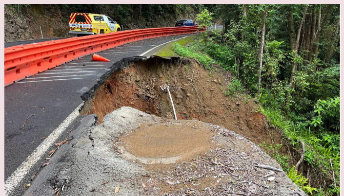
Kuranda Range Road – landslide site (February 2024)
