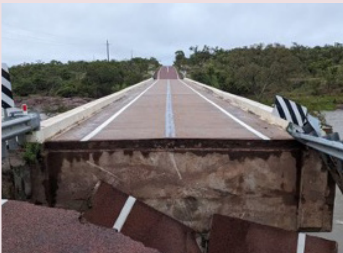
Gulf Developmental Road at Routh Creek Bridge – damage from North Queensland Monsoon Trough in January 2024 (Image: Queensland Police Service)
