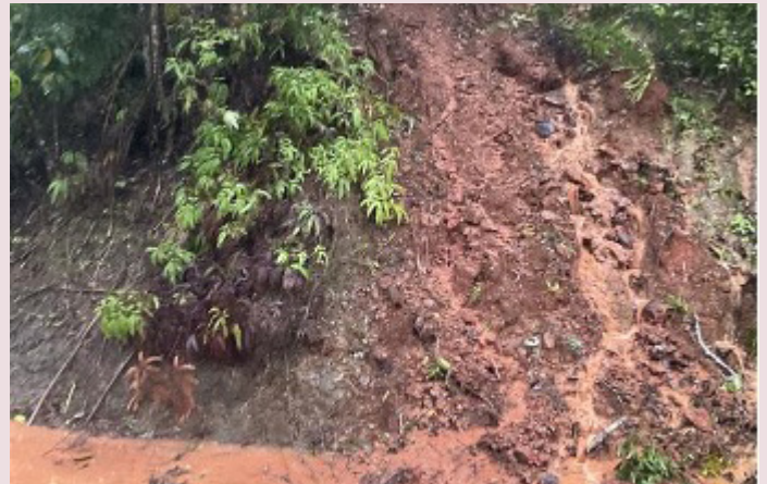
Kuranda Range Road – landslide (December 2023)
