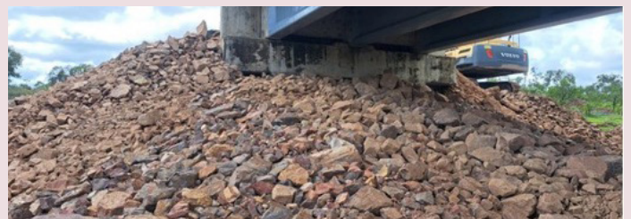
Gulf Developmental Road at Routh Creek Bridge – emergency works to restore the rock foundation around the eastern abutment (January 2024)
